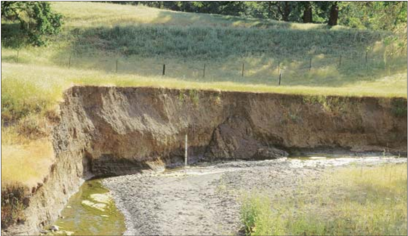
Unstable area of sediment delivery associated with bank-cutting and resulting from historical and natural influences. Current water-quality regulations require inventory and monitoring but not mitigation of this site.
